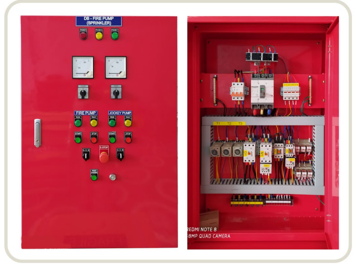
Tủ DB-FIRE PUMP
