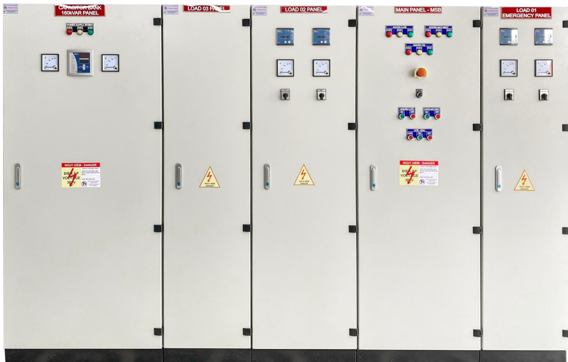
Tủ MSB 630A PANEL
