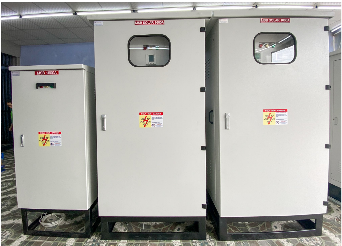
Tủ MSB SOLAR 1600A
